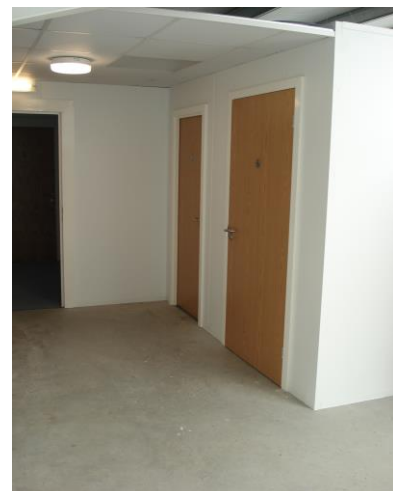
Toilet facility in office area
