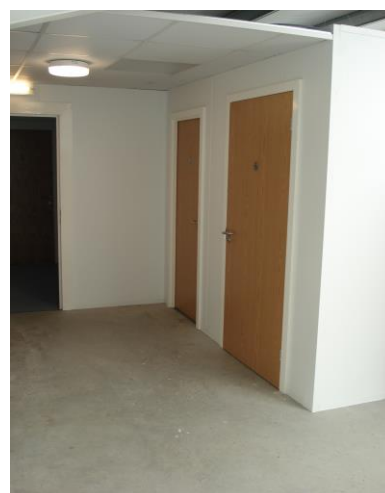
Toilet facility in office area
